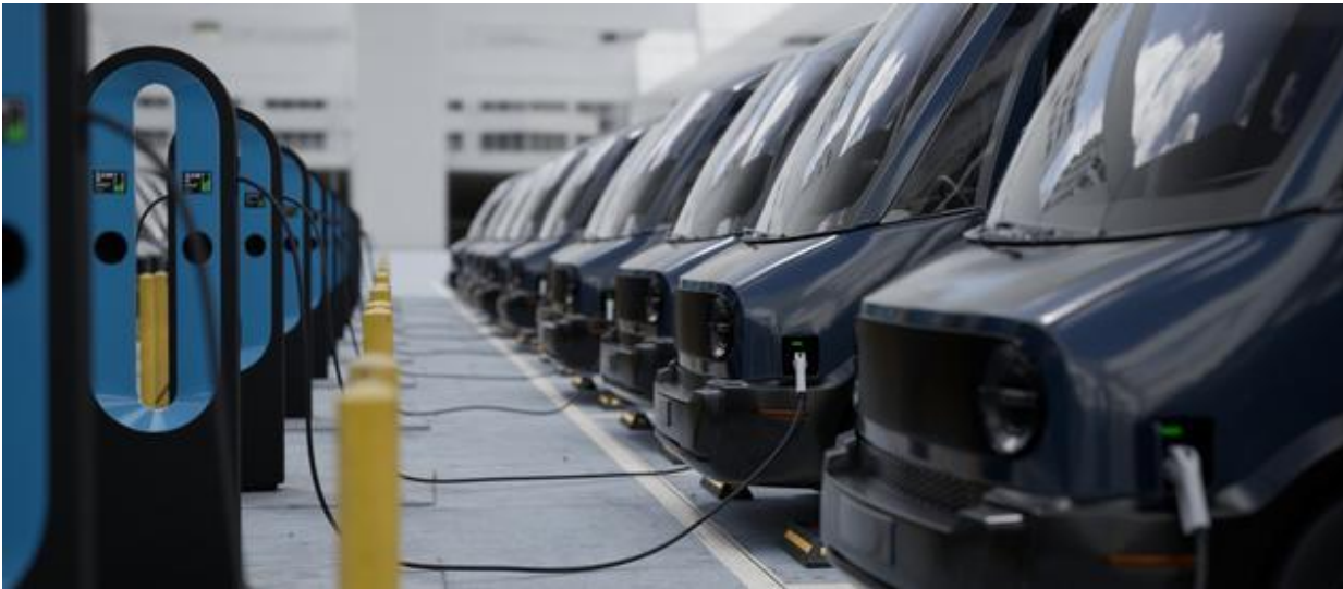
Figure 2 EV Fleet Charging
